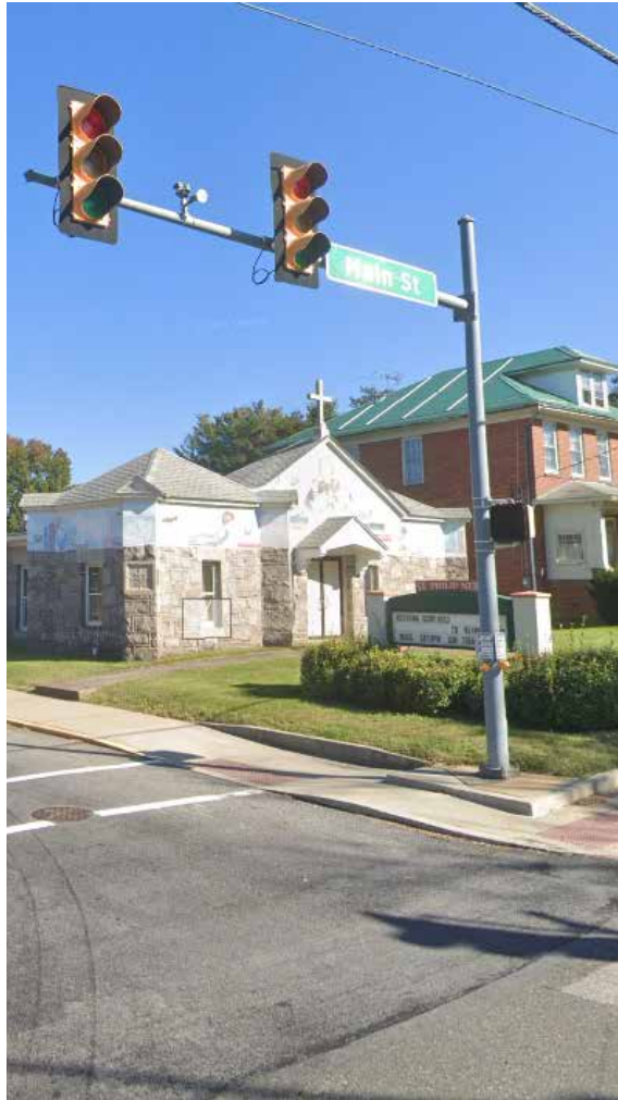
The existing traffic signal pole and support arm at Main & 6th Street is constructed of galvanized steel
