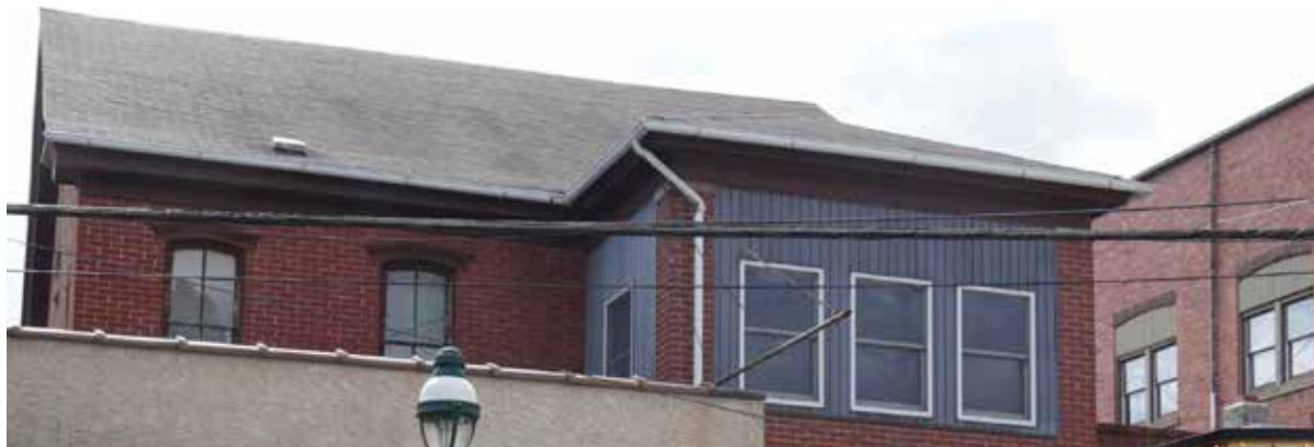
Left: the replacement windows are a similar size to the original, but the introduced siding and lack of lintel detract from the building. Right: the replacement window is significantly smaller than the original, which required filling the new void space with siding.
