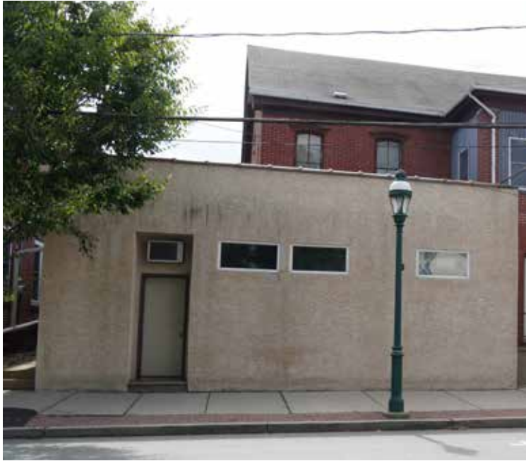
Street-facing facades should be visually interesting, with changes in colors and material. Blank walls should be avoided.
